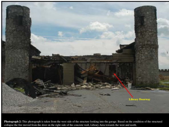
Photograph 2: This photograph is taken from the west side of the structure, looking into the garage. Based on the condition of the structural collapse the fire moved from the door on the right side of the concrete wall, Library Area towards the west and north.
