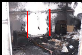
Room did not progress to full room involvement
