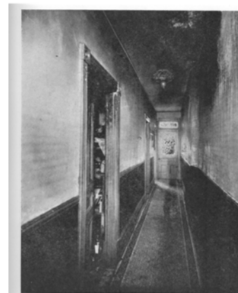
(Photograph No. 31) This picture shows a glaring example of the use of gasoline to accelerate the fire, which, however, due to lack of oxygen, extinguished itself. Note the heavy soot deposits on walls and ceiling, very little carbonizing of wood and only surface blistering from the heat.
